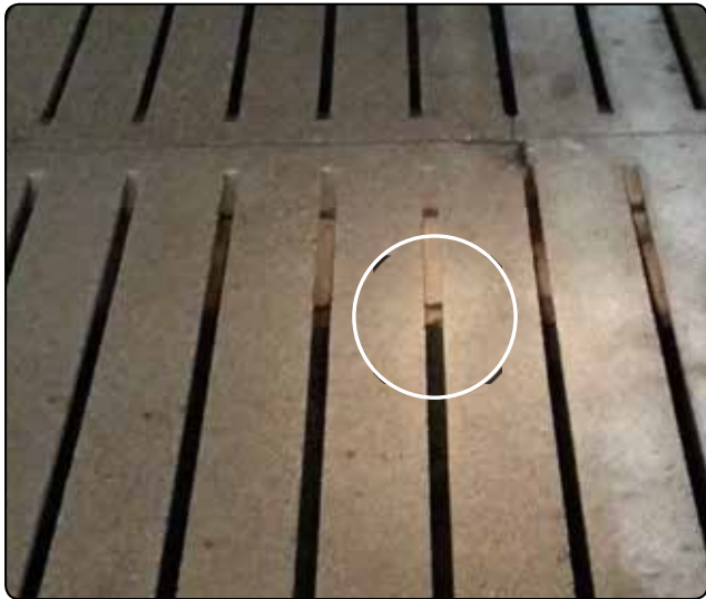
Carefully examine the support beams by shining a flashlight down through the slat openings. Look at both sides of the beams; occasionally a beam will appear to be structurally sound on one side while having rebar protruding out the opposite side.
