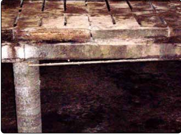
Another example of a beam with severe damage including exposed rebar.
