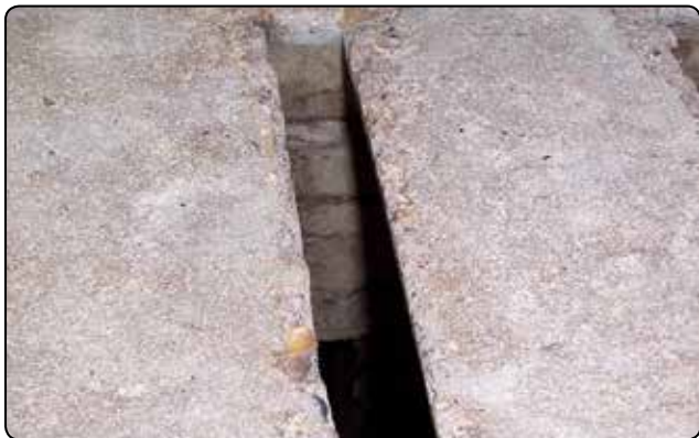
Close up view of a beam showing cracks and separation.
